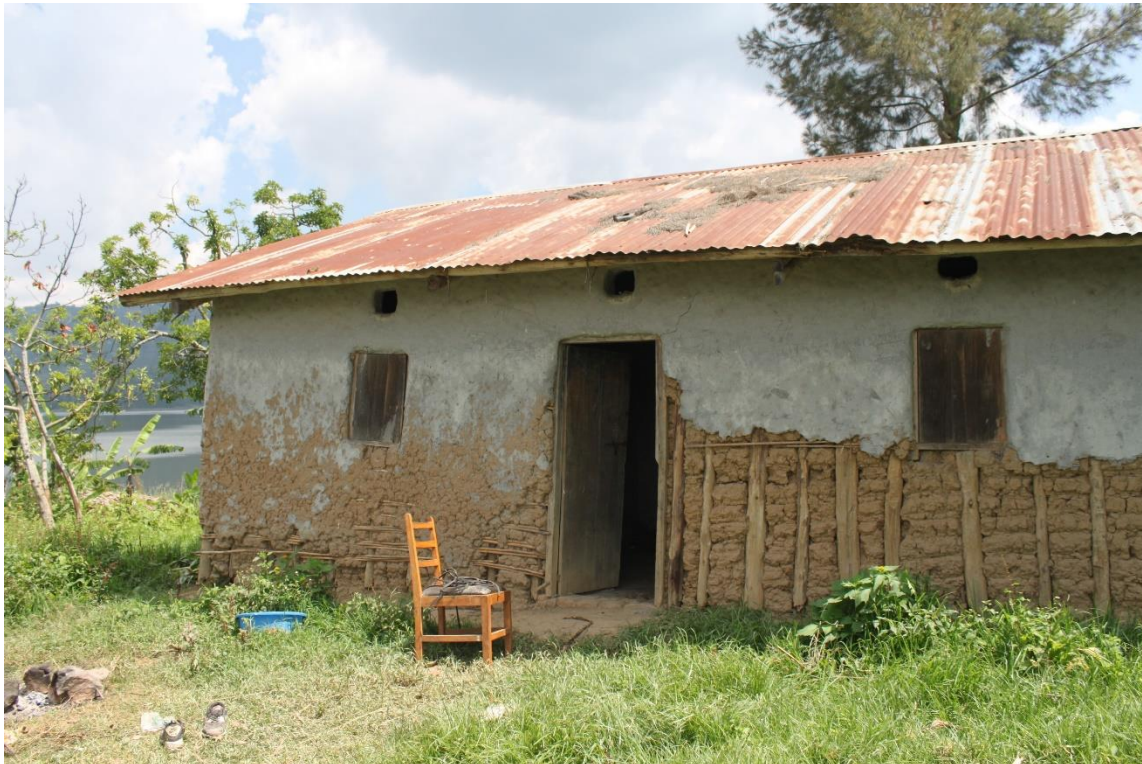
Figure 3: A Farmers house. Note the only forms of ventilation were openings near the ceiling of building
